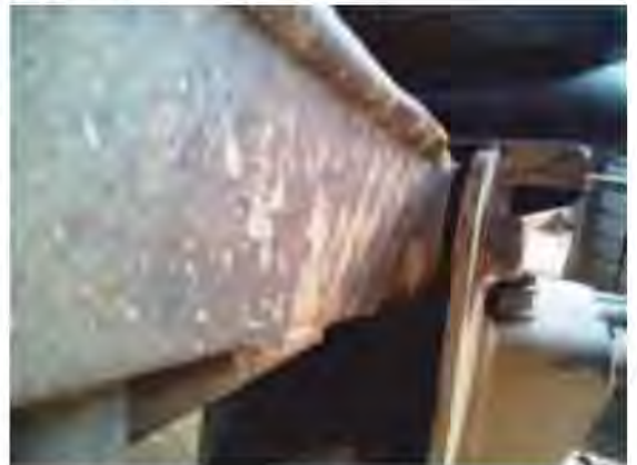
Fig. 8.2 - Incorrect (Wear Pad Missing)
